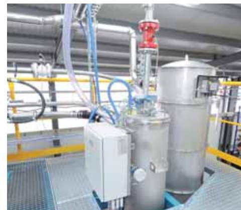
Vacuum conveyor with attached valve cabinet
