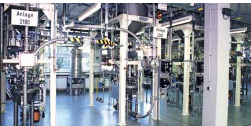
Feeding vessel conveying for chemical production
