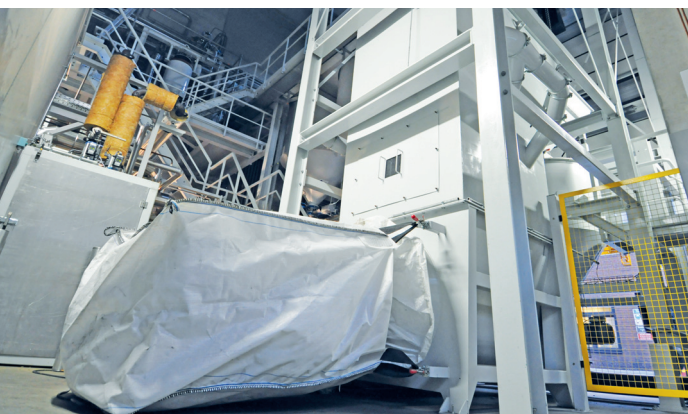
35 Big Bag compressor in automatic emptying system
