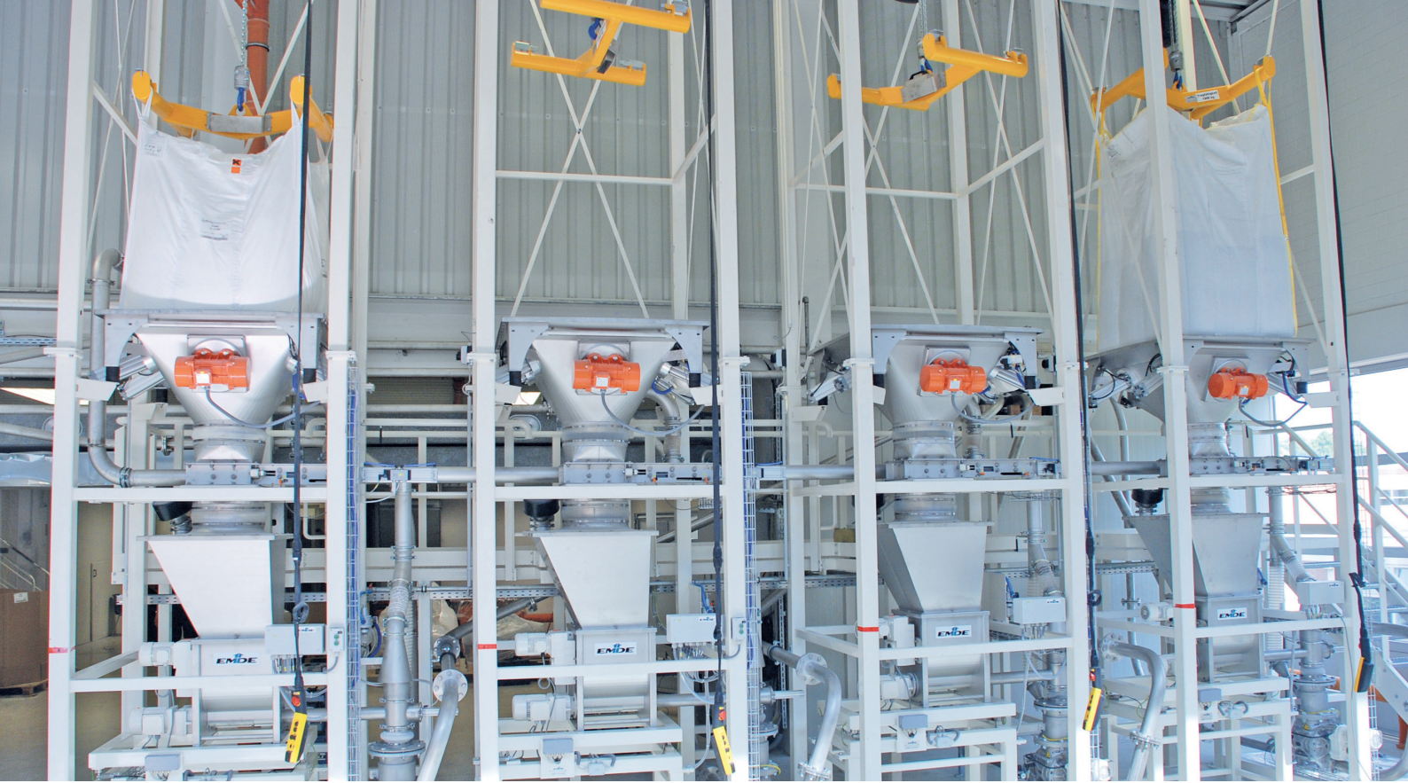
1 Big Bag emptying stations for the charging of differential metering scales
