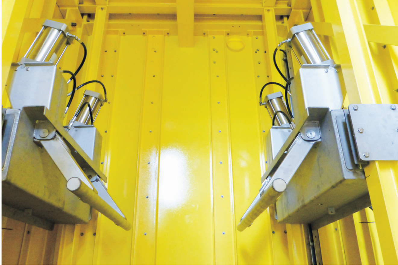
38 Side massaging device in Big Bag emptying system
