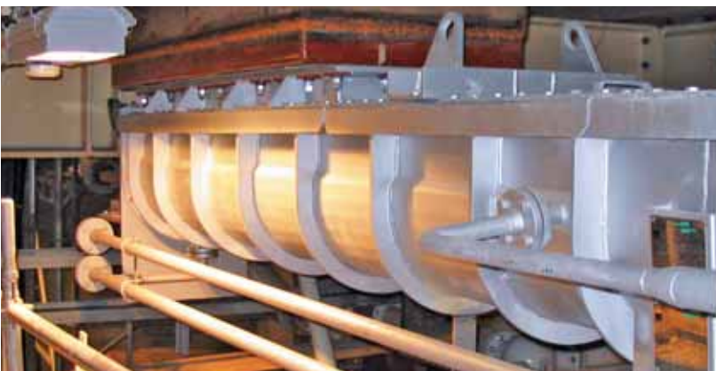
Cooling screw conveyor for ash discharge
