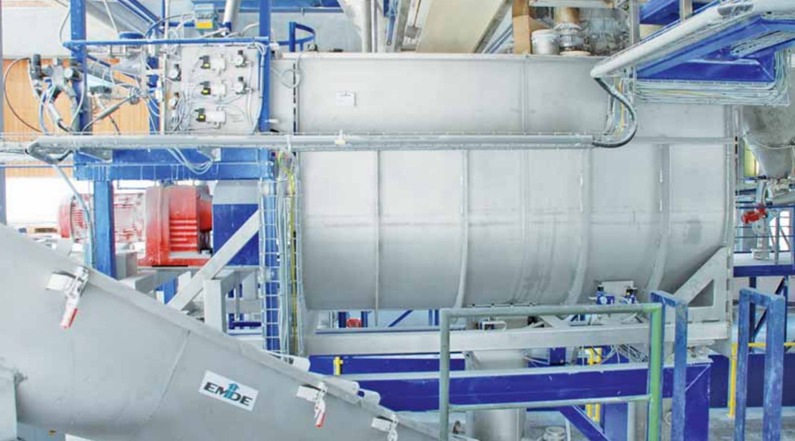
Batch mixer for sodium nitrite
