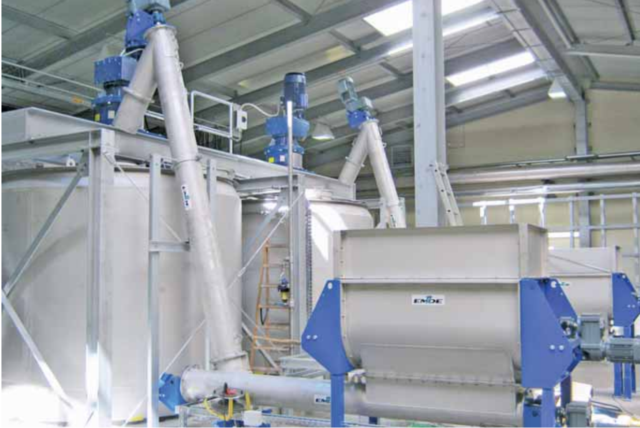
Tubular screw conveyors charging agitator vessels
