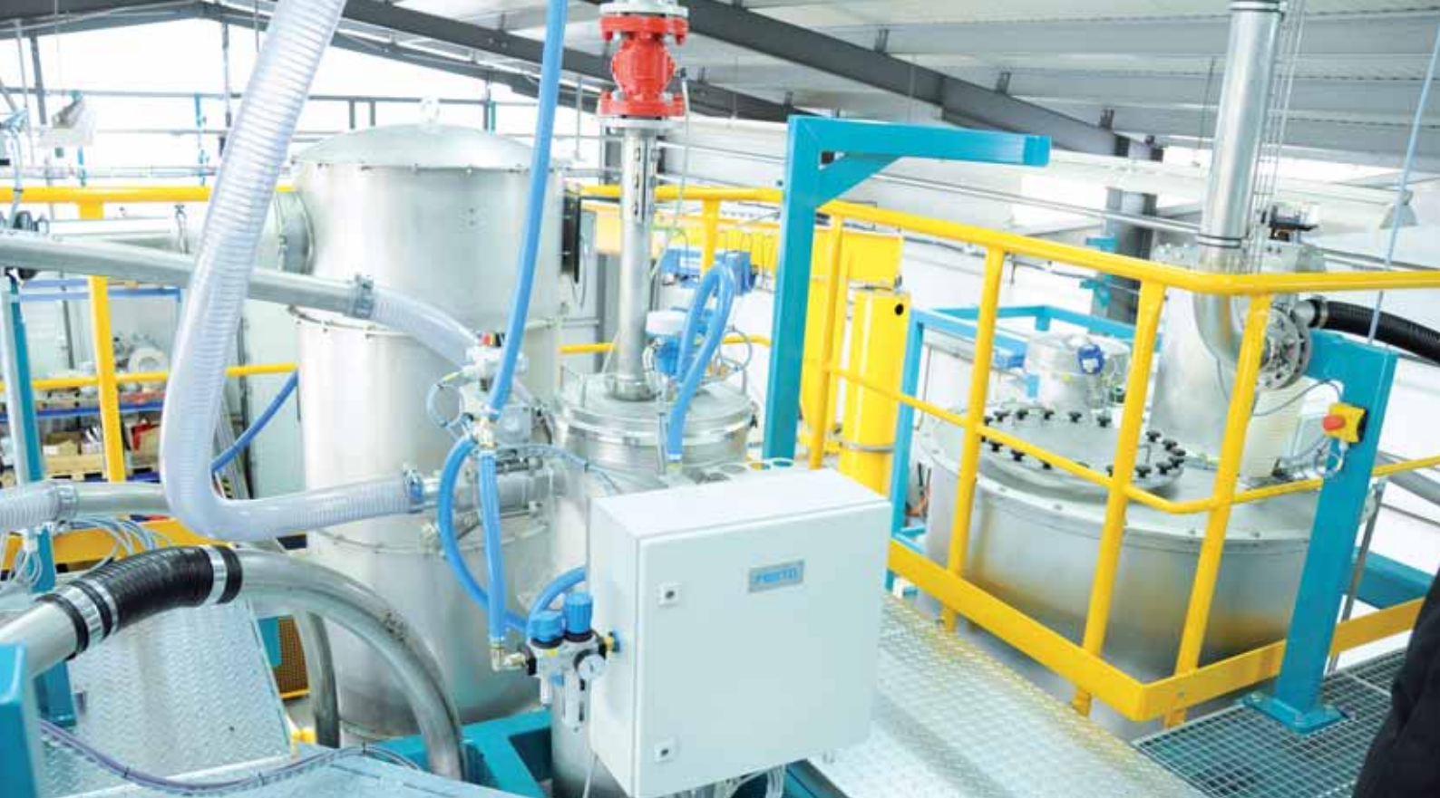
Vacuum conveyor in the technical centre system
