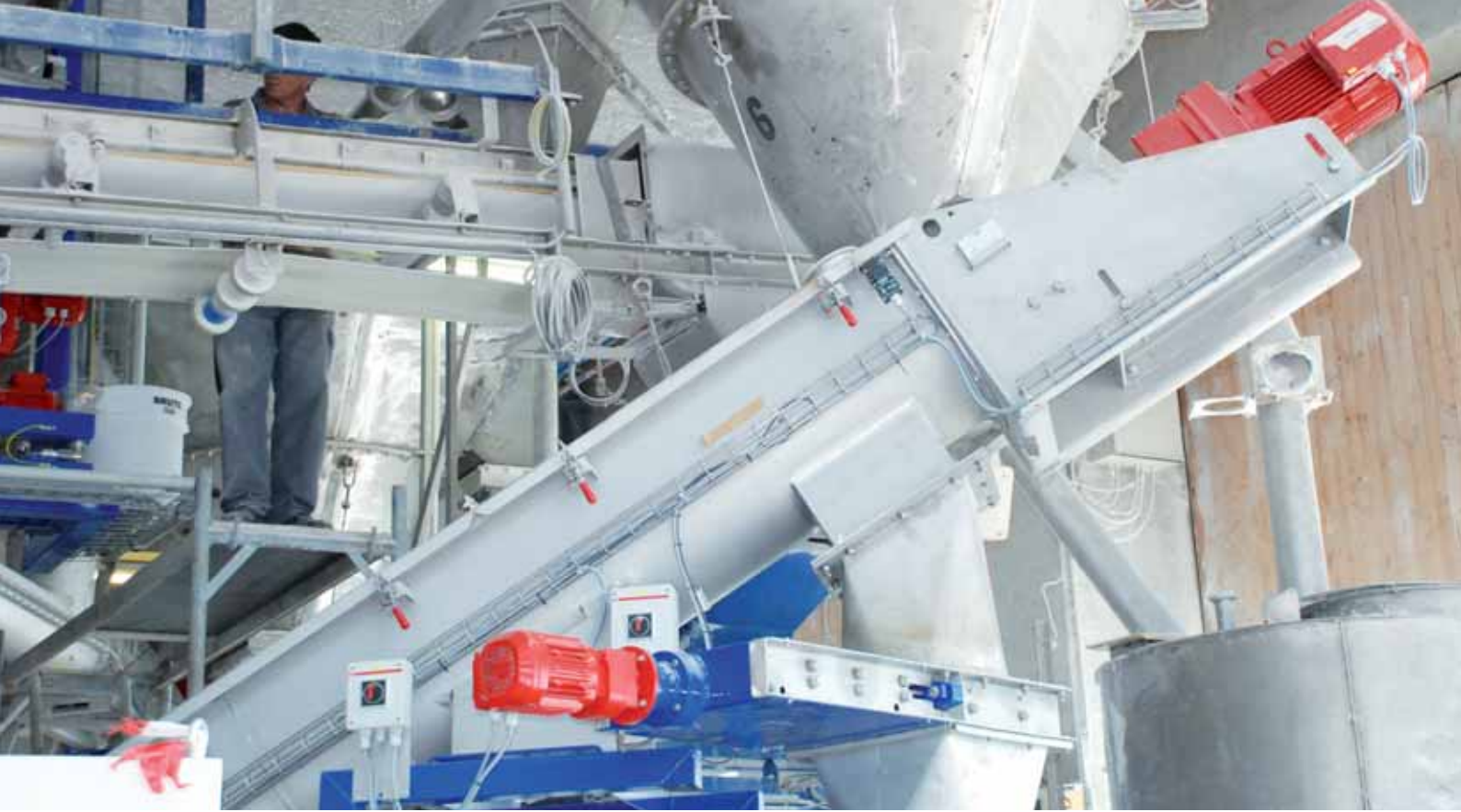
Electrically operated slide valve for sodium nitrite
