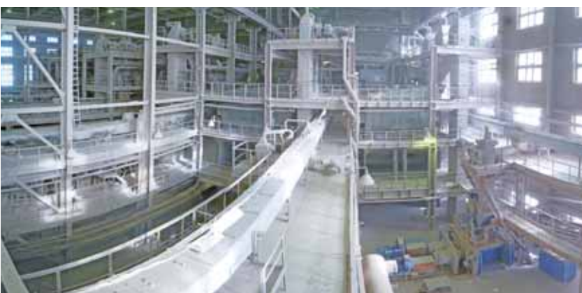
Trough chain conveyor and bucket elevators for transporting potassium salt
