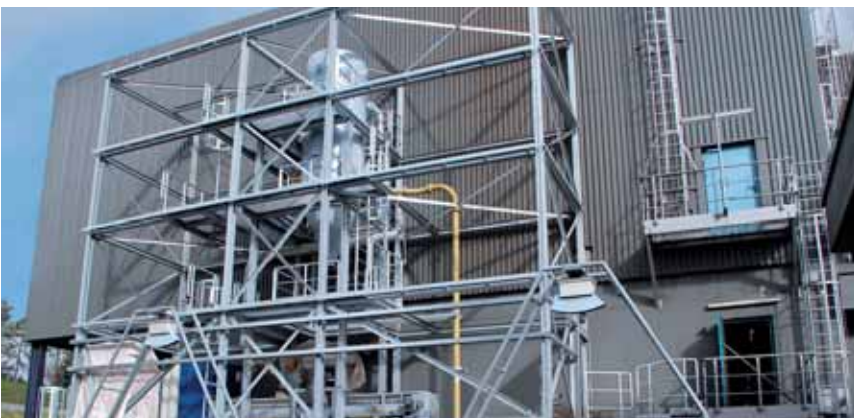
Stationary vacuum cleaning system in a lignite power station
