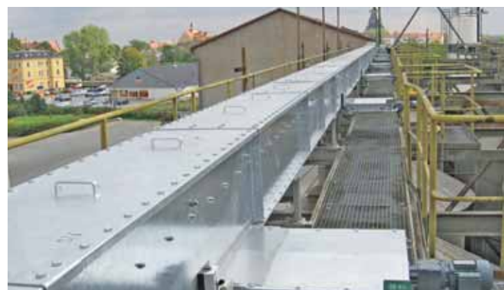
Oil seed conveying for silo filling
