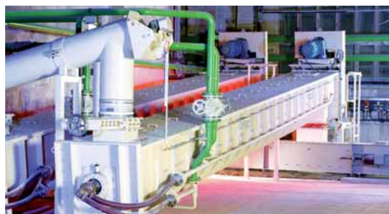
Cooling screw conveyor for soda
