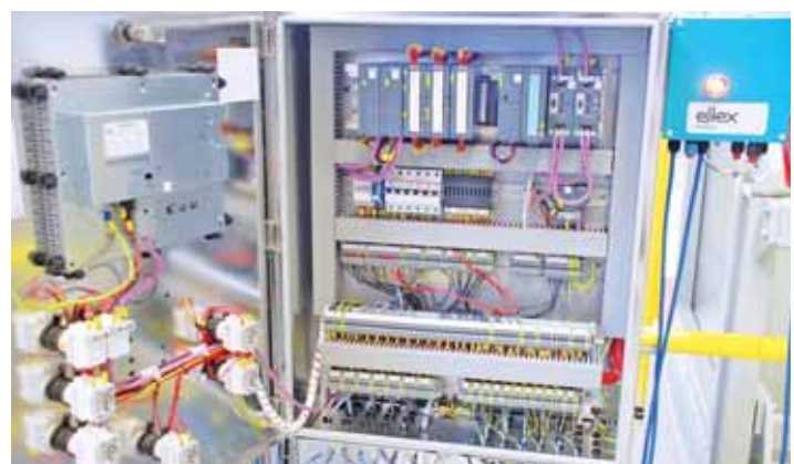
Switching cabinet interior view
